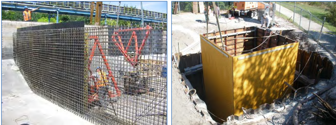
(Examples: Assembly of AGRU CPL onto wooden formwork – cast in situ applications)
